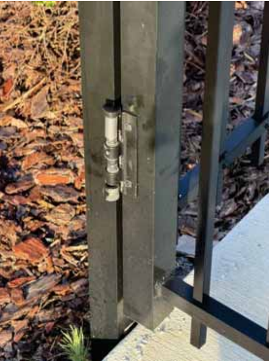
Broken Gate Hinge
